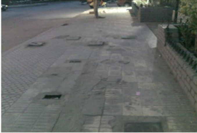
Photo (8) Metal protrusions on sidewalks
