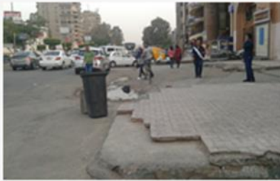
Photo (10) Damaged sidewalk; garbage bin in peoples' way
