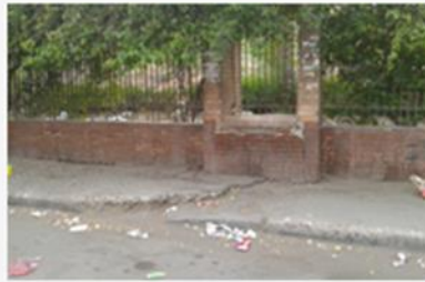
Photo (11) Wrecked pavement with non-standard height
