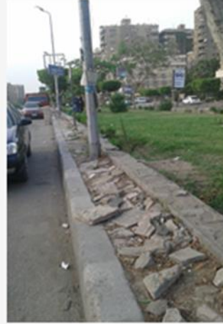
Photo (9) Wrecked pavement
