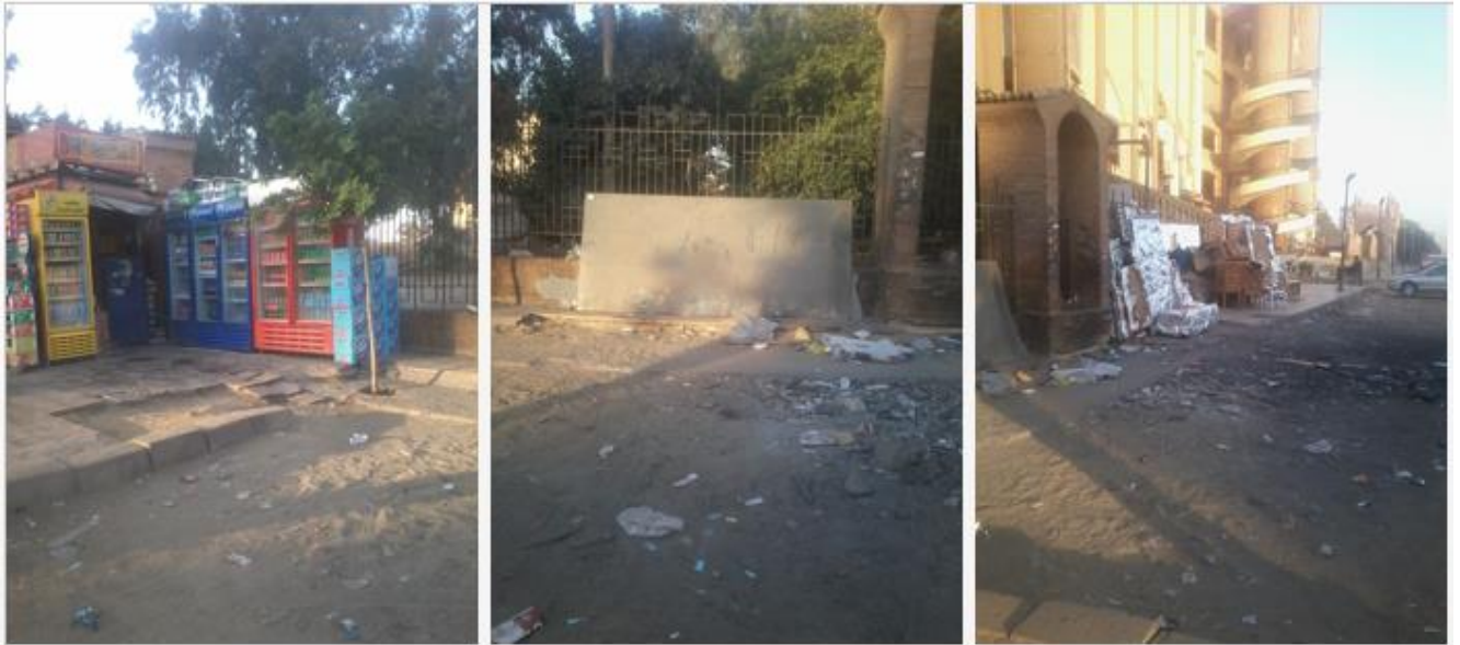
Photos (17) Encroachments on pavement
