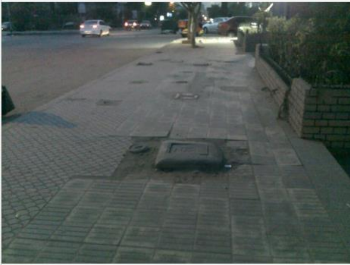
Photo (4) Metal protrusions on the pavement.
